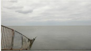
Seaside of the dike, Groningen coast. [2]
